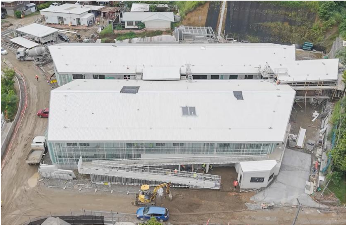
Photo 3 – The Naha Birthing and Urban Health Centre is close to completion, with the carpark and road works now underway.
